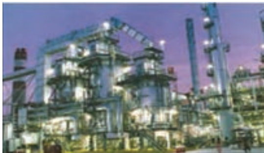
A. 1 Water purification
