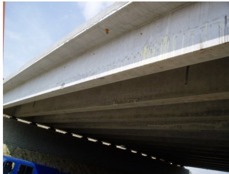
Figure 28. Overall view of the repaired crack
