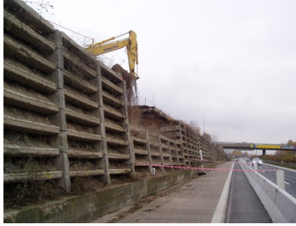
Figure 16. Original state of the retaining wall
